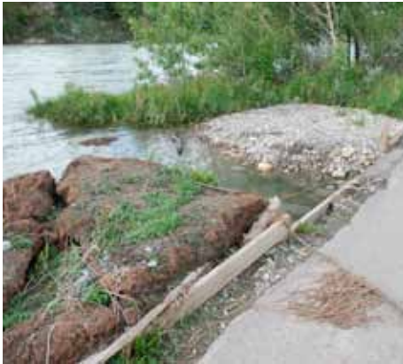
Culvert requiring replacement
